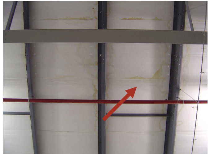
Moisture condensation can accumulate in fiberglass over time. First becoming visible as simple water stains.
