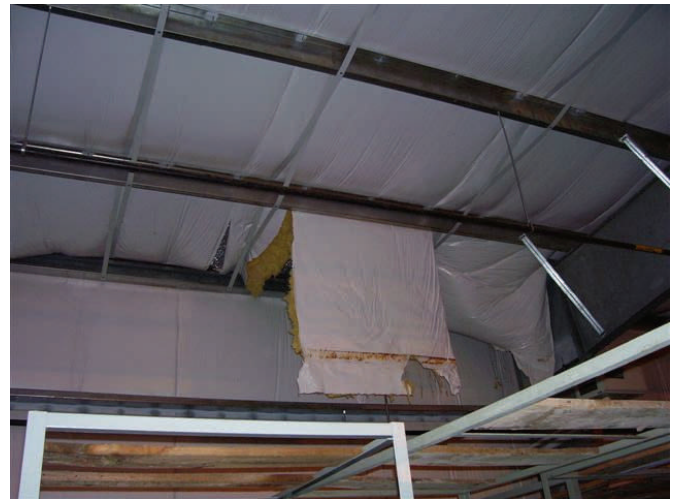
As the moisture accumulates over time it causes the fiberglass to sag, then fall out of place as the weight becomes too great. Since the fiberglass has a vapor retarder facing, the moisture cannot escape. As it accumulates it decreases thermal performance.
