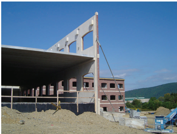
Structural beams are cast into the walls to support the precast floor planks.
